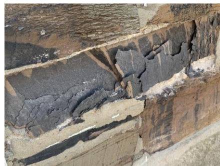
Concerning stone deterioration on the southern side of St Peter's
