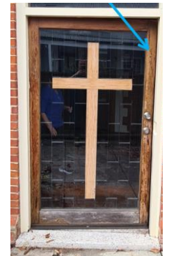
Wood rot evident
